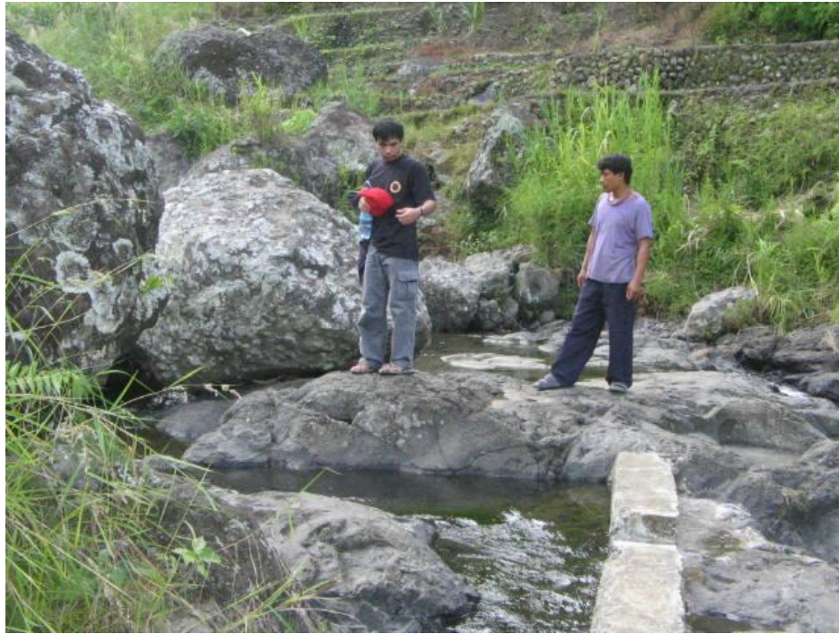
Engr. Galera Inspecting the condition of the weir of the micro hydro project.
